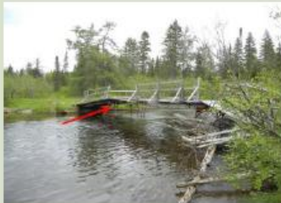
View of dilapidated bridge at Mt. Carleton
